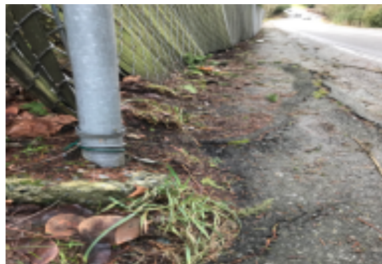
Figure 1.3 Exposed concrete base is a tripping hazard.
