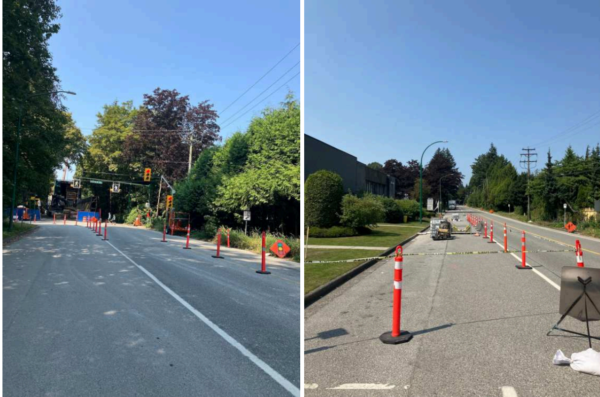
Figure 1: Sharing the lane on Winston St. Left: Single-lane alternating traffic along Winston St. This works for people driving, but is extremely uncomfortable for people cycling and potentially dangerous if followed by a person driving aggressively. Right: The construction site on Winston St. unnecessarily takes away all road space for people riding bikes and forces them to share a narrow lane with vehicles.
