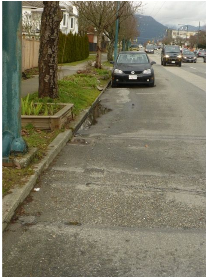
Figure 3 - Nanaimo Street drainage issues at Ferndale
